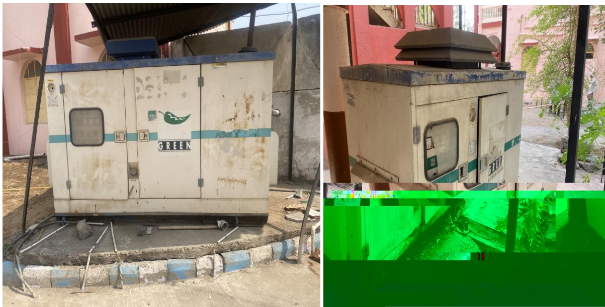
Figure: - DG set College premises
